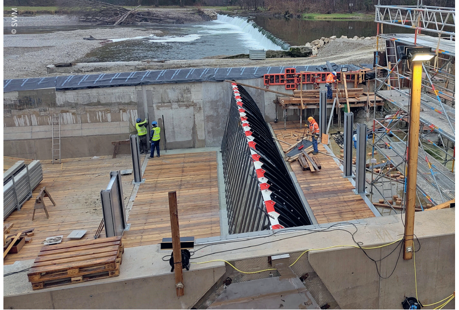
Installation work on the pneumatically operated flap gate system, supplied by British industry specialists Dyrhoff UK Ltd.
